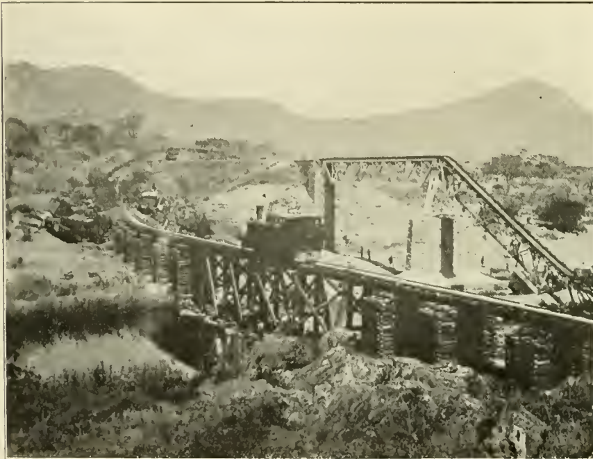
TEMPORARY TRESTLE, AND DESTROYED MAIN LINE BRIDGE, KAAPMINDEN, SOUTH AFRICA.
